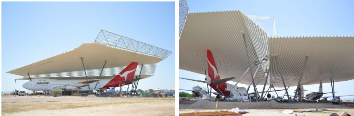
Qantas Founders Museum Airpark Roof with Aramax Roof Sheeting complete. Photo taken February 2020.
